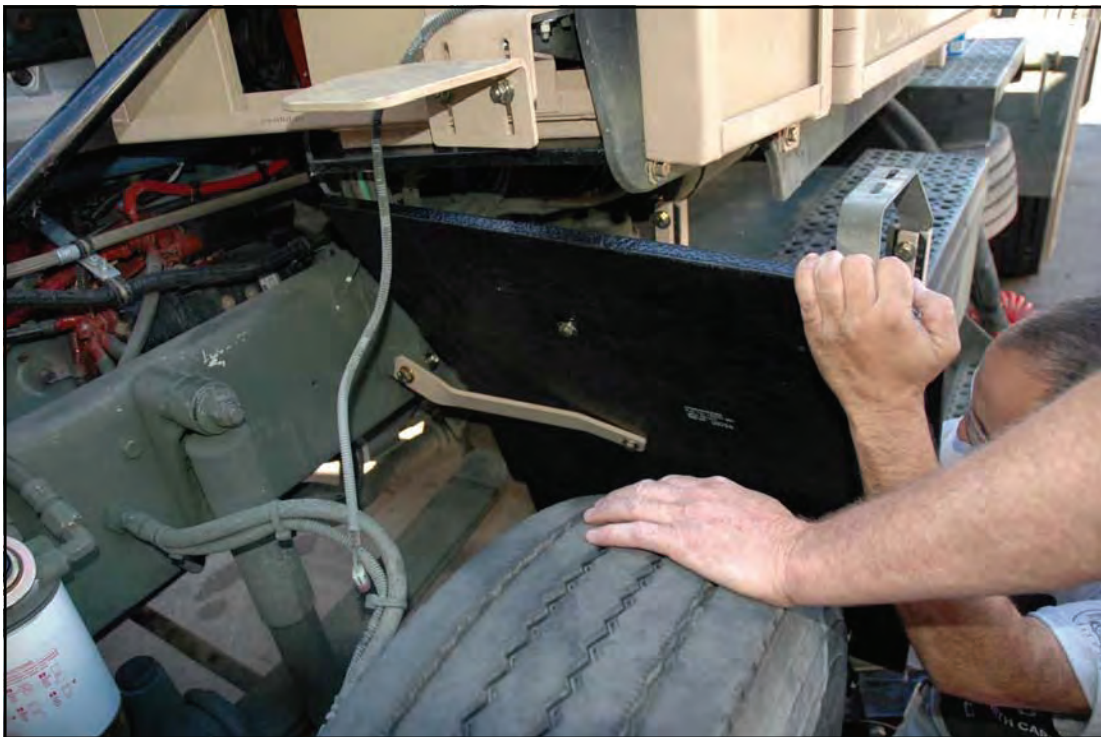
6.) Attach P/N 110-324-001 to the front of the truck's wheel well underbody support frame.
